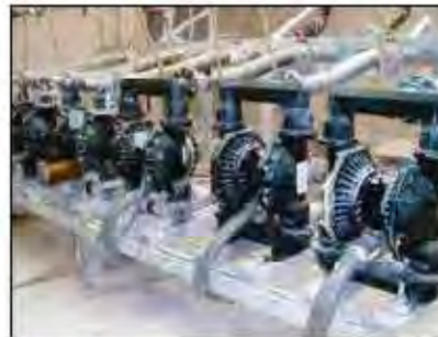
3" diaphragm pumps mounted on a skid to transfer clay in a ceramic manufacture
