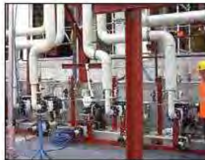
2" stainless steel diaphragm pumps assembled with PVDF pulsation dampeners used to download hydrofluoric acid
